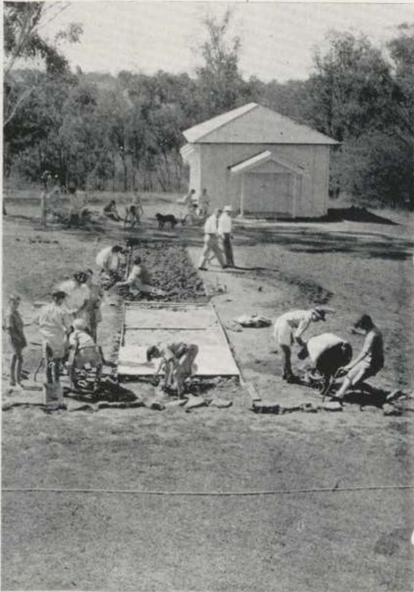
"Operation Canterbury" in action. Laying the path leading to site of Memorial.
